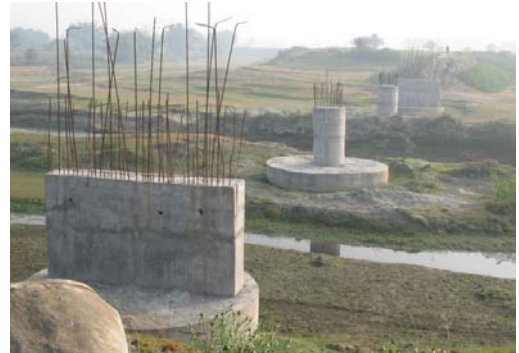
Budhikhola Bridge as on 5/12/2007. It was expected to be completed on 15/11/2004.
